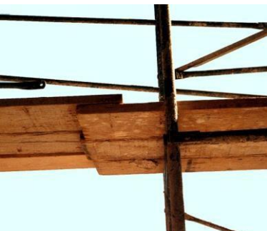
Planks not properly overlapped
