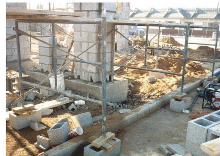
Inadequate support –In danger of collapse?
