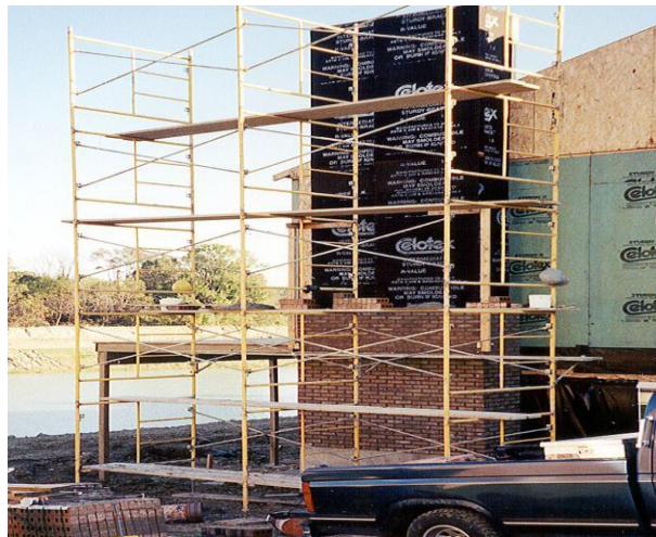
This is not a properly constructed scaffold
