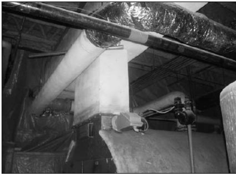
Pipe and boiler insulation
