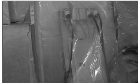
Isolated electrical panel
